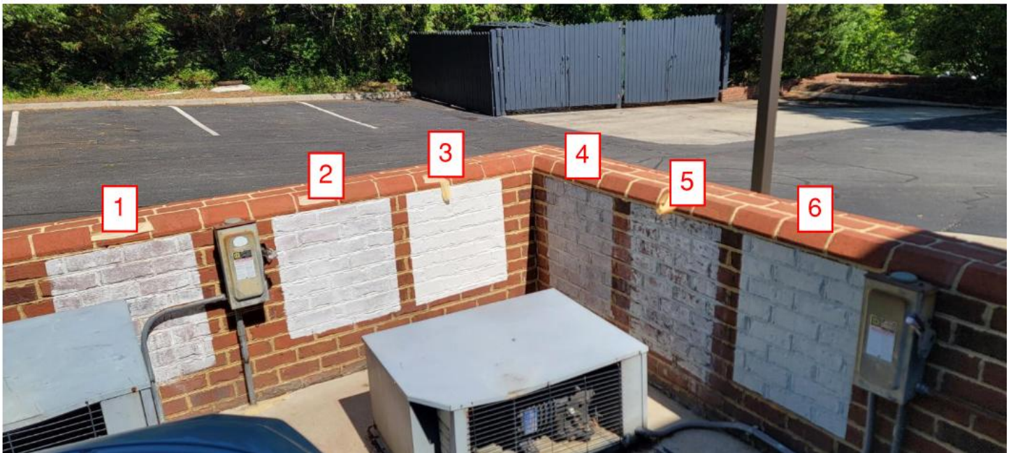
Figure 1: Staff photo of the applicant's lime wash samples on the inside of the mechanical screen behind the Crozet FasMart store (May 12, 2026).
